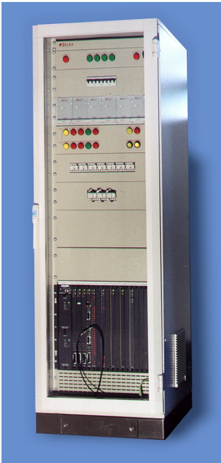
The steam generator water level control system, cabinet
